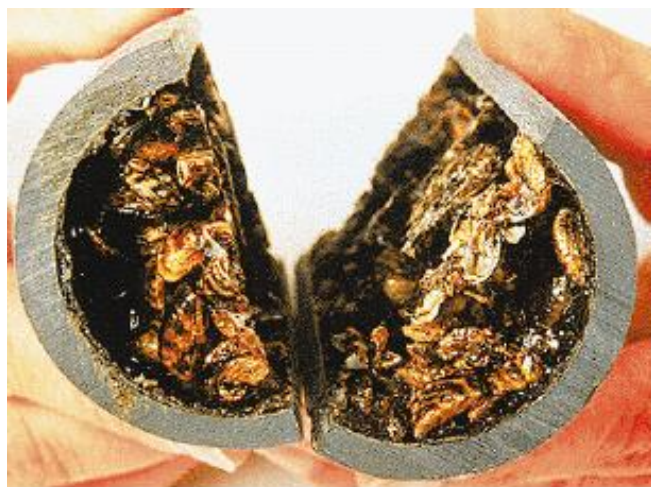
Figure 2. A pipe clogged by zebra mussels (provided by Peter Yates)
